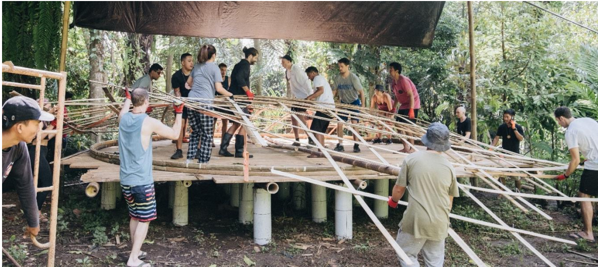
Figure 7. Assembly, bending, and popping up of the grid (Bottom: Jumpa Zoe, March 2023, © Bamboo U)
